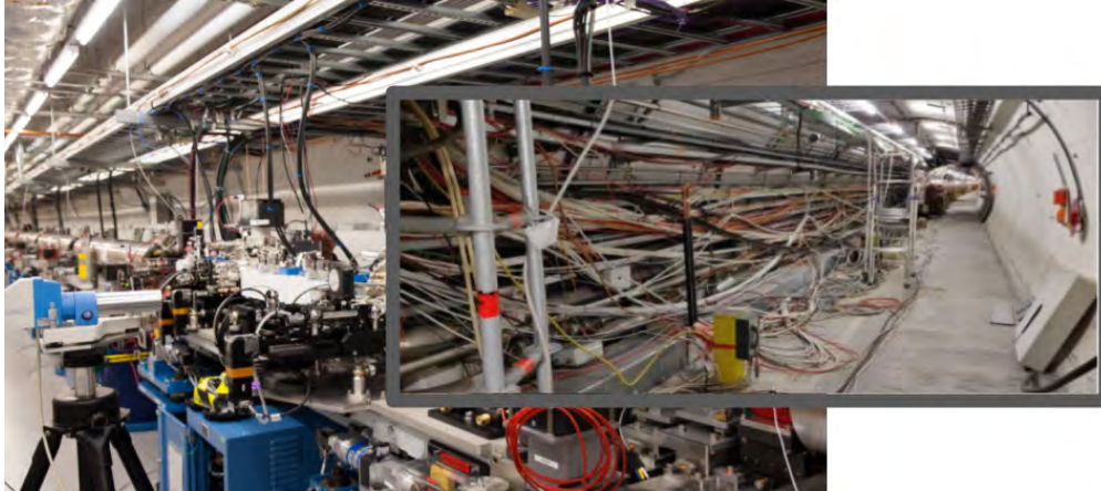
Figure 19: Examples of current “cable salads” impacting facility spaces and operational flexibility.
