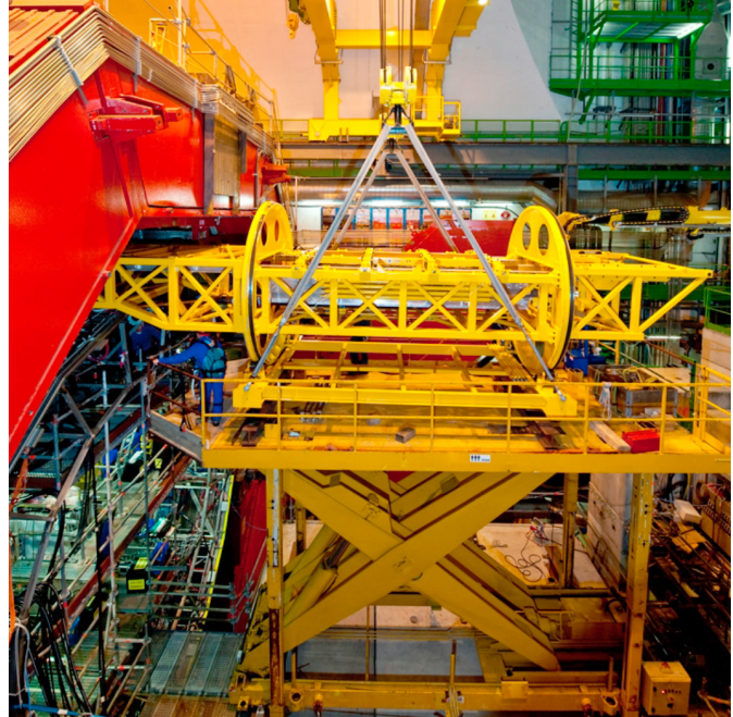
Figure 7.3: View of US-led ALICE ElectroMagnetic Calorimeter (EMCal) modules during installation in the ALICE experiment; one of the 10 EMCal modules, weighing over 7 tons, is being inserted.
