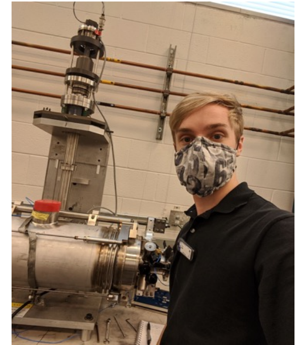
C100 cavity tuner drive mechanism behind and above cavity.
