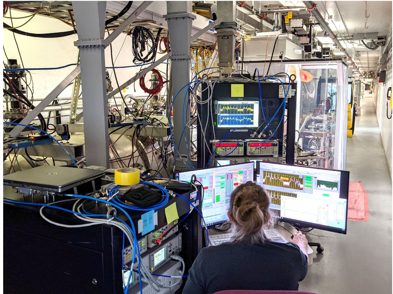
Two of 4 channels of the RF system in the tunnel.
