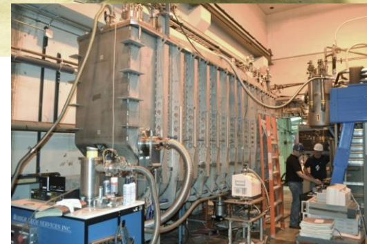
2014 ATLAS Energy and Intensity Upgrade Cryomodule
