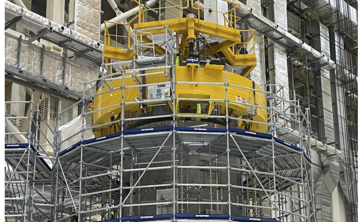
The third module has been centered on the central solenoid assembly stack.
