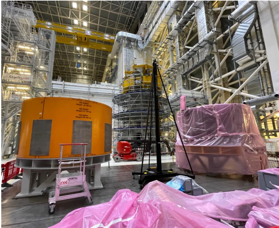
Central solenoid magnet assembly is underway inside the Assembly Hall. From left: magnet test load, module stack, and fourth module for stack
