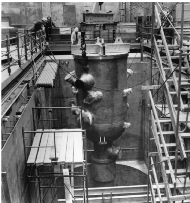
FIGURE A1.4. Original Installation of the HFIR Pressure Vessel. The HFIR building and pool were designed to support pressure vessel replacement.
