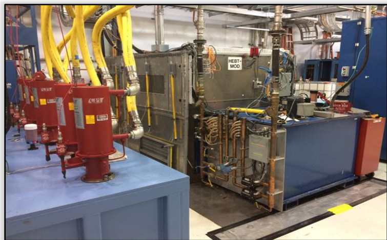
RF high voltage modulator undergoing heat test
