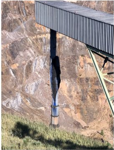
The rock is very abrasive on distribution systems
