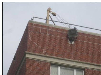
Spedding Hall Deteriorating Brick/Limestone Exterior (circa 1953)
