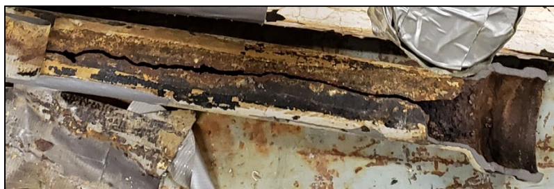
Spedding Hall Deteriorating Sewer Piping (circa 1953)
