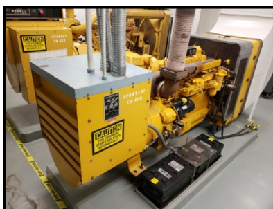
Harley Wilhelm Hall Backup/Emergency Generator (circa 1970)
