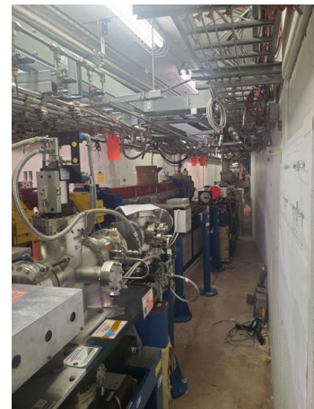
Fig. 5: View inside the storage ring tunnel with a new magnet module visible in the back.
